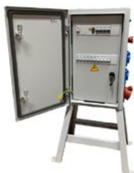
Coffrets de distribution
